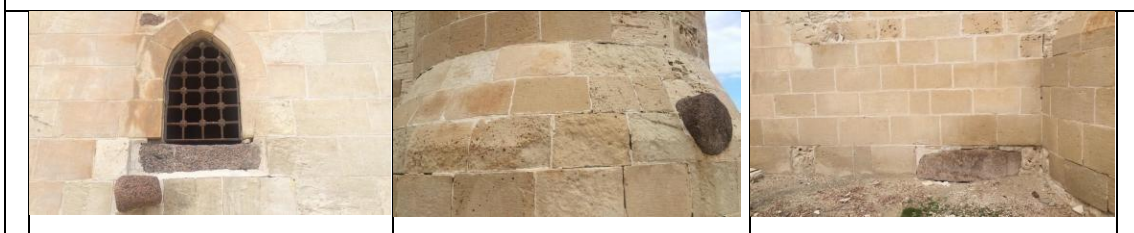
Fig. (12) The photographic elevation of some details of the main tower of the citadel.
